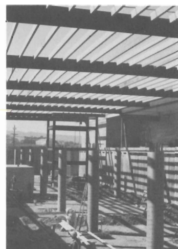
Expansion of Stanford Plant's Building 1 will allow growing space. Solid State group will move into new area early in 1967.
